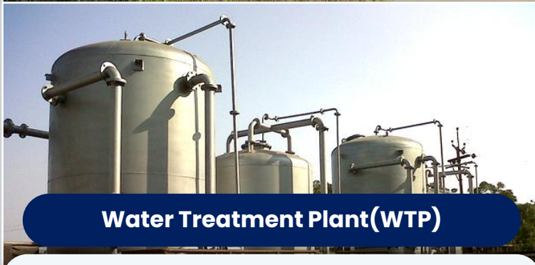
Pre-treatment Clarification & Pumping System
